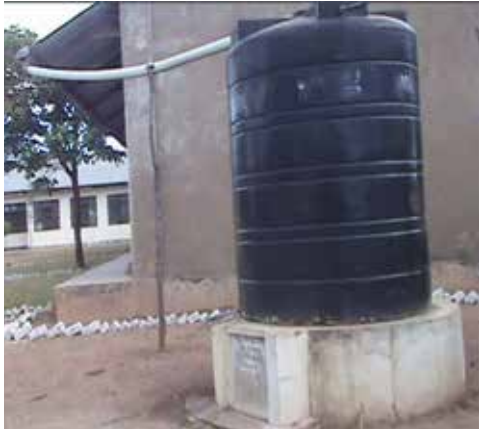
Rain water harvesting from Kabungu Secondary School roof top, Mpanda district, Katavi region
