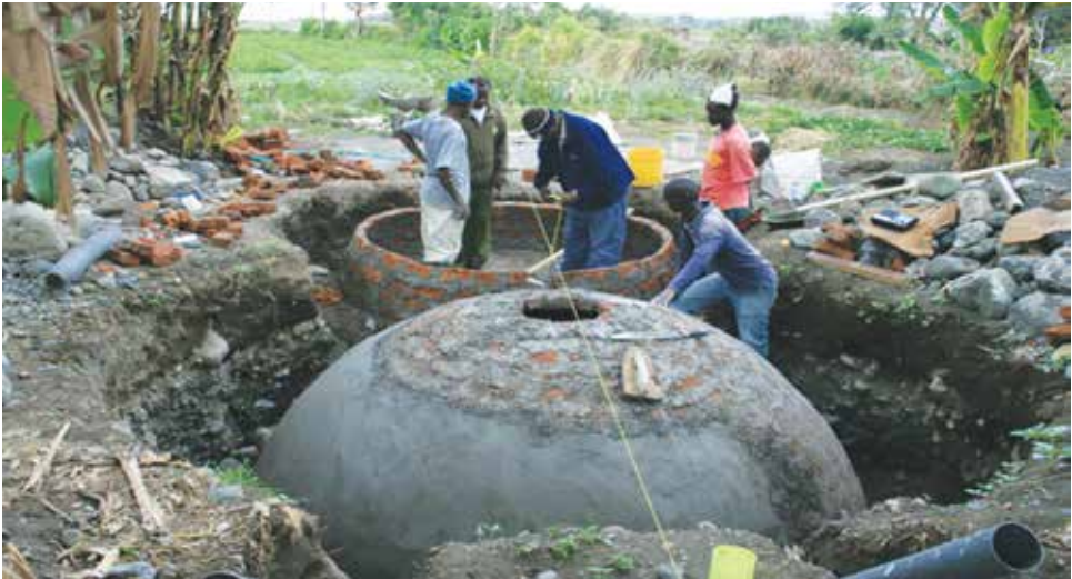
Example of biogas production plant in Kilimanjaro
